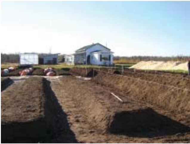
Constructing the permanent raised beds. Piles of wood chips and bags of leaves waiting to be placed in the alleys and on the beds, respectively.
